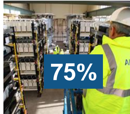
Alstom Grid UK HDVC Power Systems
