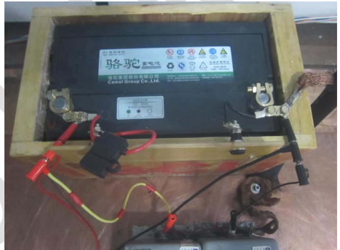
Picture for battery side
